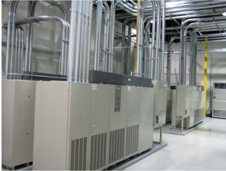
UPS Room (Contains many UPS Batteries)
